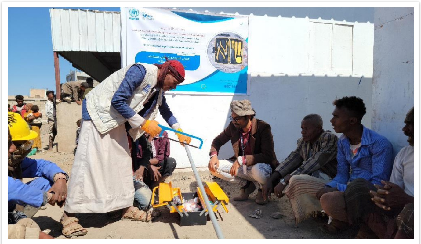
IDPs at the Al-Judad site in Dhamar Governorate received a plumbing box as part of the UNHCR-funded SDF-CCCM site maintenance project activities. All needed to maintain and repair the water points and latrines on the site are contained in the plumbing box. A brief description of the box's contents and how to utilize it was provided by a plumbing expert on the site. The community committee will be in charge of the plumbing box on 21/12/2022. pic taken by M. Almutawakel CCCM site coordinator
