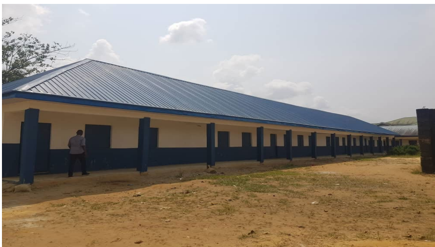
Government Secondary School Ikot Effanga: - Construction of new school building. @UNHCR/Aluka Christopher
