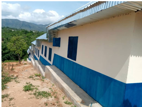
Border Community Secondary School Amana, Obanliku LGA, CRS (New construction of one Block of 5 Classrooms and Staff Offices.) @UNHCR/Aluka Christopher
