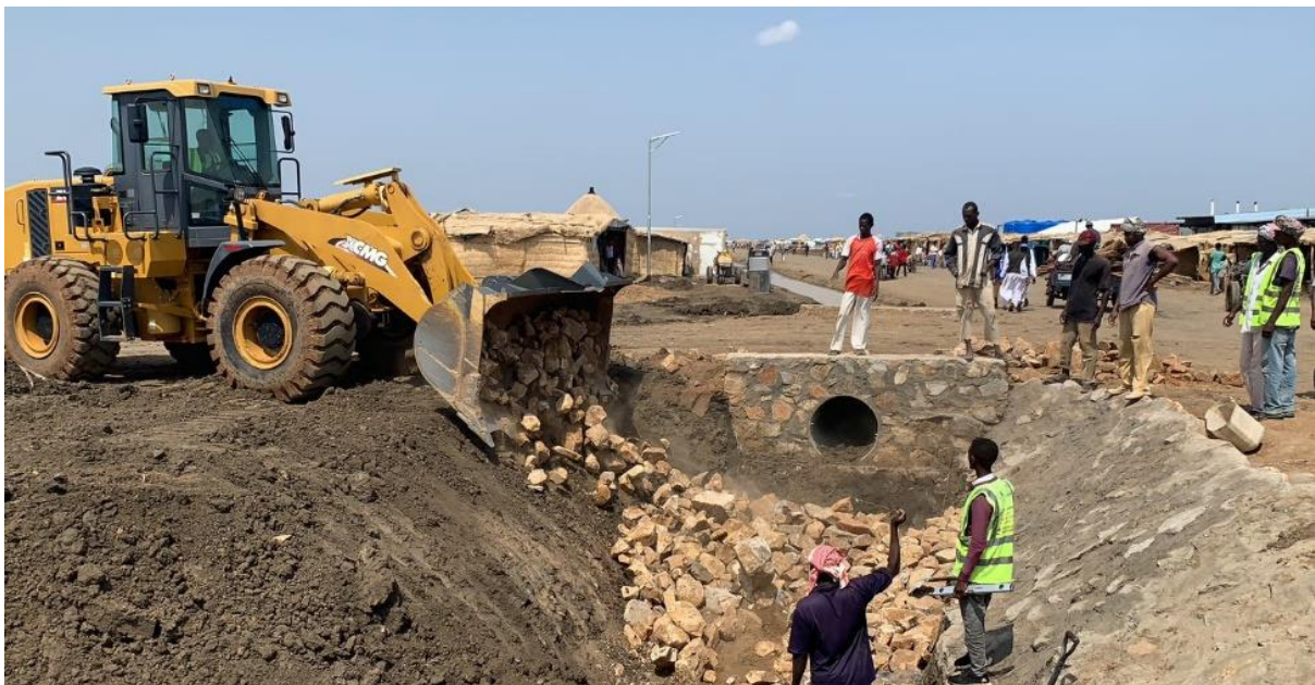
Drainage construction as part of a joint UNHCR/WFP project which is currently ongoing in Tunaybah and Um Rakuba.
