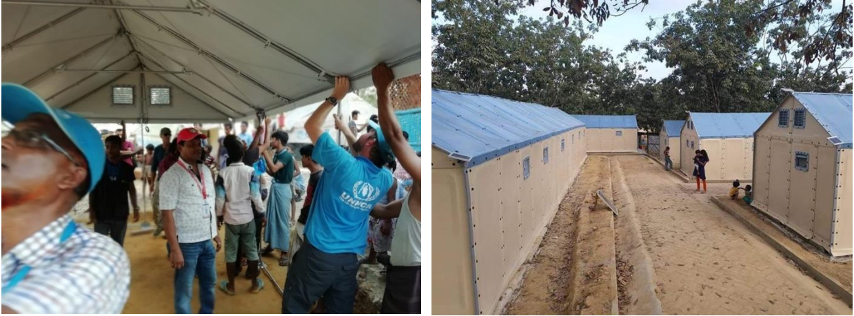
Refugee Housing Units go up in UNHCR's reception centre adjacent to the Kutupalong refugee settlement. Each unit takes over four hours to erect. © UNHCR/S O'Brien, K Shahnam
