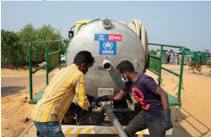
UNHCR works with multiple partners, as well as more than 500 WASH volunteers to maintain water, sanitation and hygiene standards. UNHCR has established thousands of communal latrine facilities; the fecal sludge from these facilities is treated in one of the fecal sludge treatment plants. @UNHCR/ Kamrul Hasan
