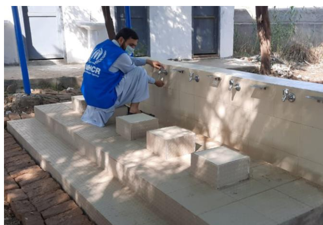
As part of UNHCR's COVID-19 response, water, sanitation and hygiene facilities are being improved in support of refugees and host communities across Pakistan. UNHCR recently completed such work in Ghulam Banda refugee village in Khyber Pakhtunkhwa. © UNHCR/J. Khalid
