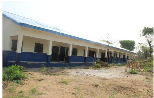
School block of six classrooms constructed by UNHCR in St Peter's Primary School, Adagom (Ogoja LGA, Cross River State) / ©UNHCR / L. Agjende/2019
