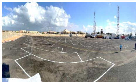
The asphalt platform at Ras Jdir border entry following rehabilitation works. © UNHCR
