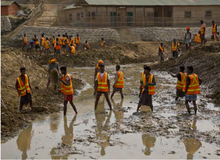
Construction worker volunteers supported by UNHCR and partners play an important role in improving the infrastructure in the camps, including bridges, stairs, pathways and roads. Refugee volunteers work relentlessly to improve the lives of the community each day. (UNHCR/ Caroline Gluck)
