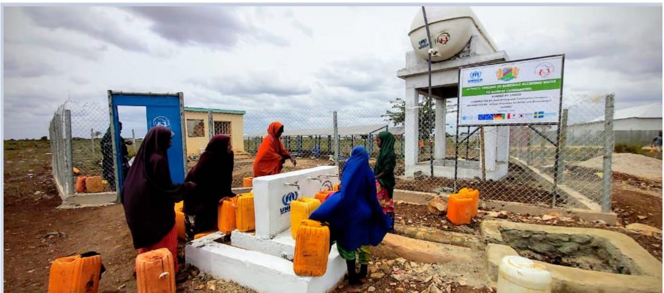
Access to clean water is essential in the fight against COVID-19. UNHCR has constructed two boreholes in Baidoa, Somalia that are accessible to more than 3,000 internally displaced families. UNHCR Somalia.
