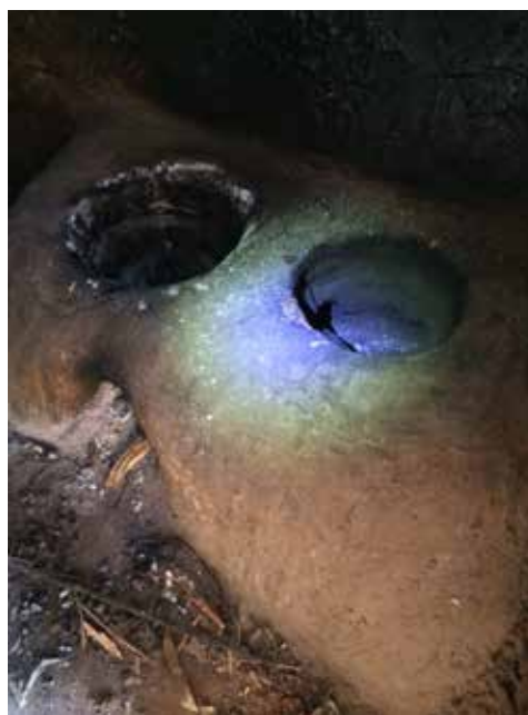
Chimney opening of a household clay stove.
