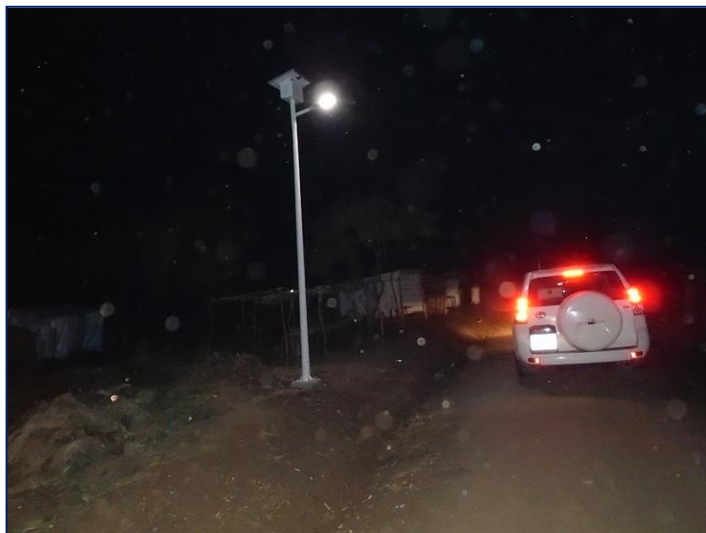
Bidibidi Settlement, additional solar street lights are being installed in Zone 2 for improved safety and security, Nov 2016. UNHCR/S. Dzikunu
