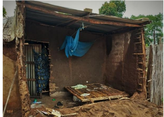
Refugee house destroyed in Maratane settlement, Nampula Province. ©UNHCR/Irene Omondi
