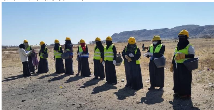
Labors working on site- installing latrines, rehabilitation of water distribution in Dhamar photo© UNHCR
