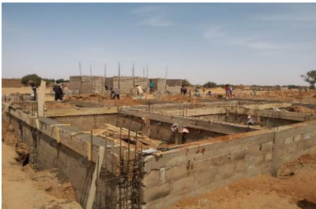
Construction of the new Health Center (CSI type II) in Abala, supported by the EU Trust Fund
